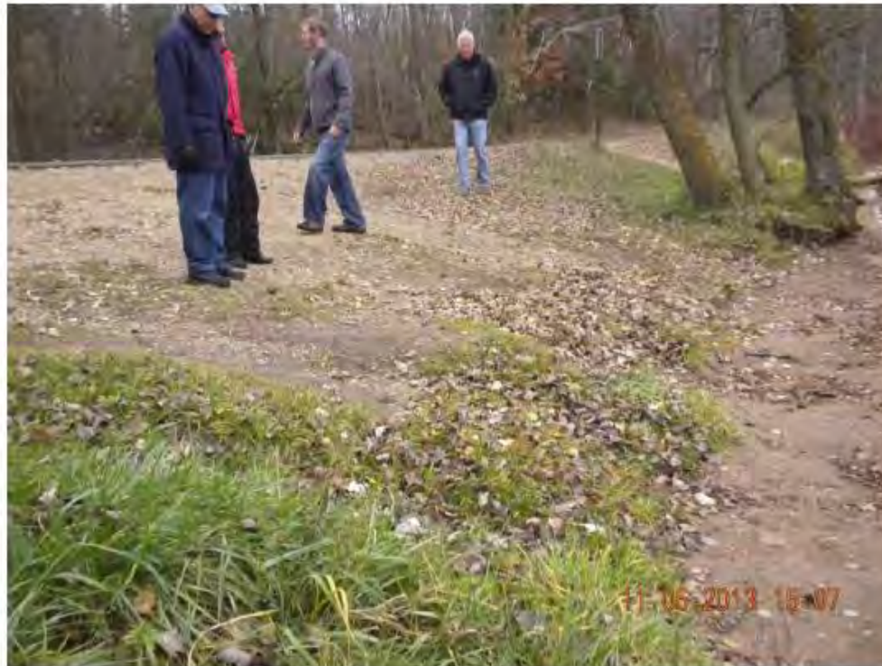
Erosion at Church Pine Boat Landing (in Town of Alden right of way)
